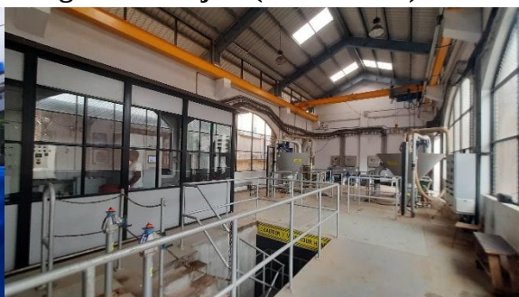
Bambalapitiya Pumping Stations
