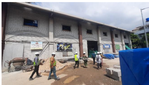
Thimbirigasyaya Pumping Stations
